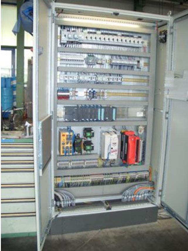
Electrical cabinet in hybrid technics : PSS / S7-300
