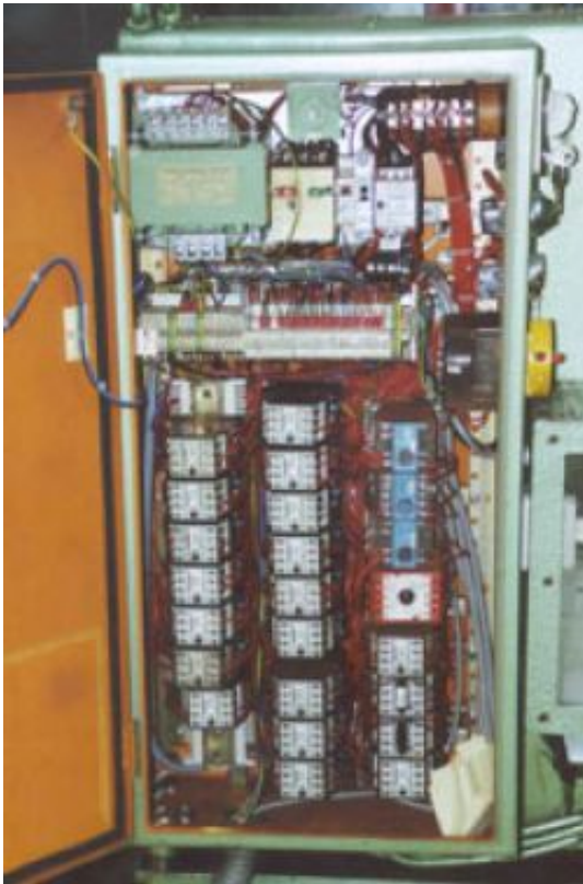
Electrical press cabinet in obsolete technique
